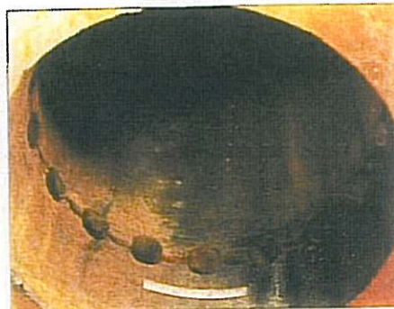
Fig. 2 — The circumferential through-wall crack in tube row number 4 is apparent along the inside surface of the header.
