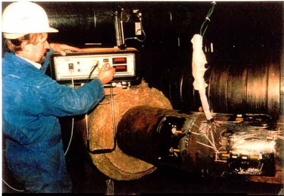
Fig. 13. Calibration and baseline data recorded prior to re-insulation and piping system start-up.
