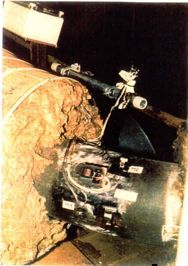
Fig. 11. Typical installation of capacitive strain gages on surface of main steam pipe.
