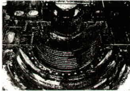
4. Lower casing is shown after repair and addition of new partition in steam inlet area
