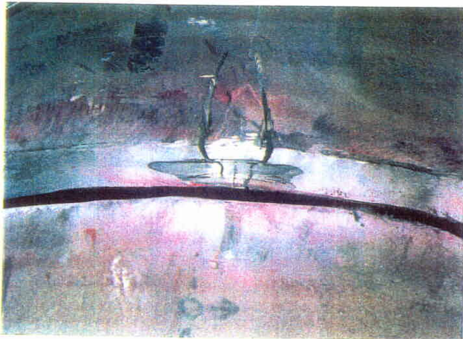
FIG. 5. VIEWS OF TRANSVERSE CRACKS AT BOAT SAMPLE NO. 2.
